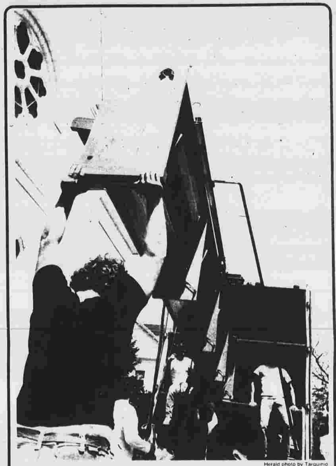
Workers from an Ohio-based company unload one of 50 new pews that have been installed at St. James Church this week as part of a major renovation project. The renovations, scheduled to be completed soon, were required to bring the 110-year-old Catholic church at 896 Main St. up to code, said Father Francis Krukowski.
